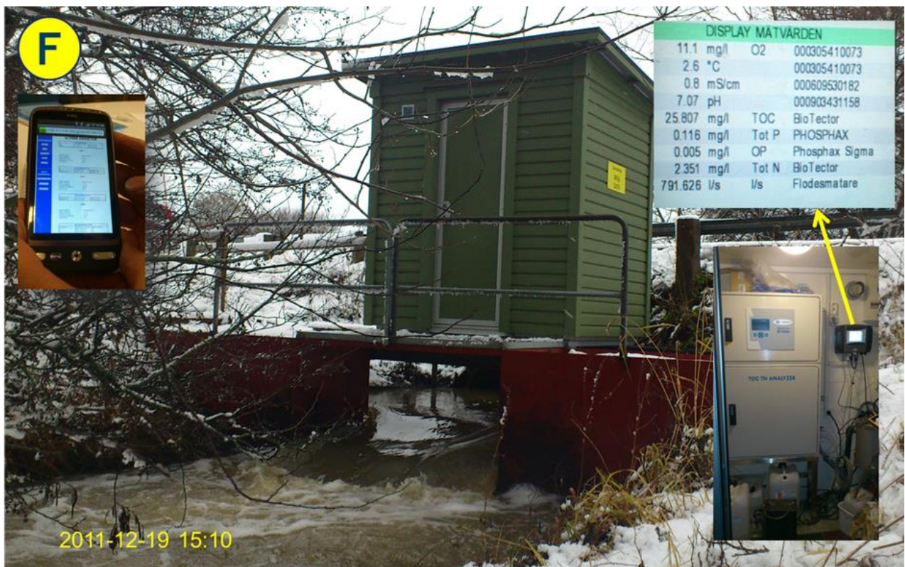
Figure 9 Swedavia measurements in reference point "F" measuring important water quality parameters and water flow [Norling 2011]
